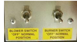
BLOWER SERVICE SWITCH
