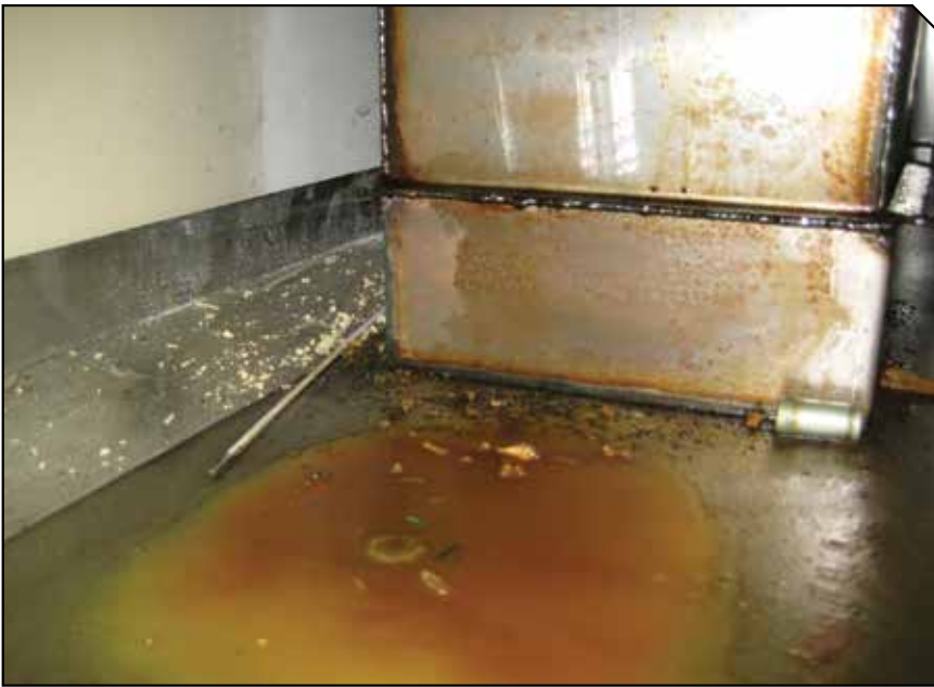
FIGURE 2. Grease pooled on top of hood from leaking duct.
