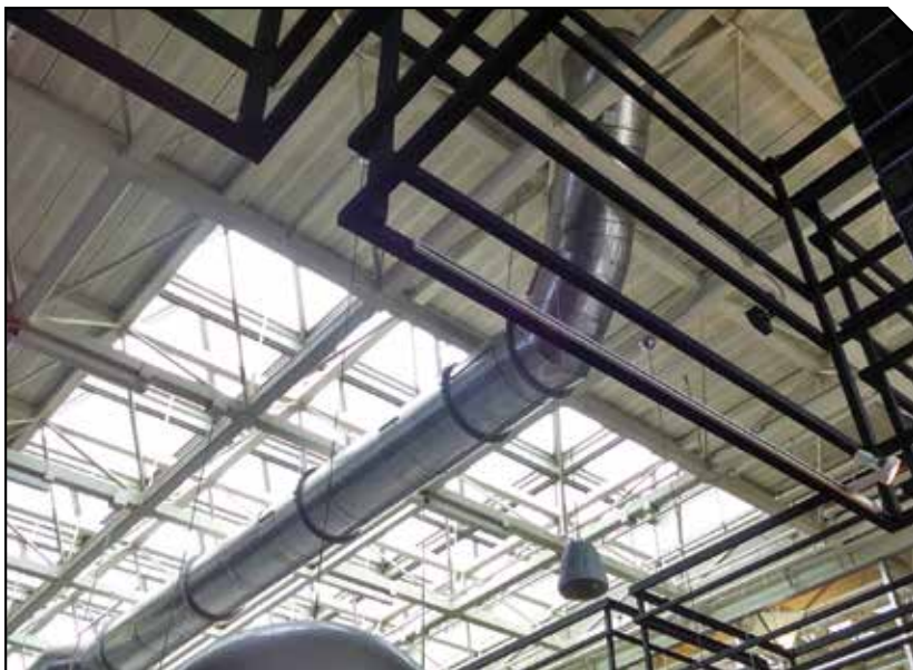
FIGURE 5. Listed duct installation for airport restaurant.
