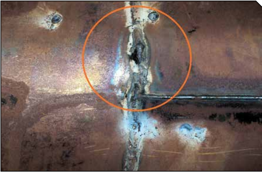
FIGURE 1. Fire scene photo showing unlisted duct with noticeable holes in welds.
