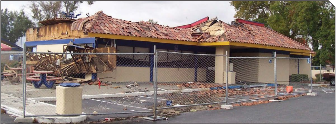
FIGURE 2. The fire was not suppressed because fusible links were encrusted with grease.
