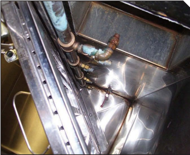
FIGURE 3. Hood plenum with automated hood cleaning.
