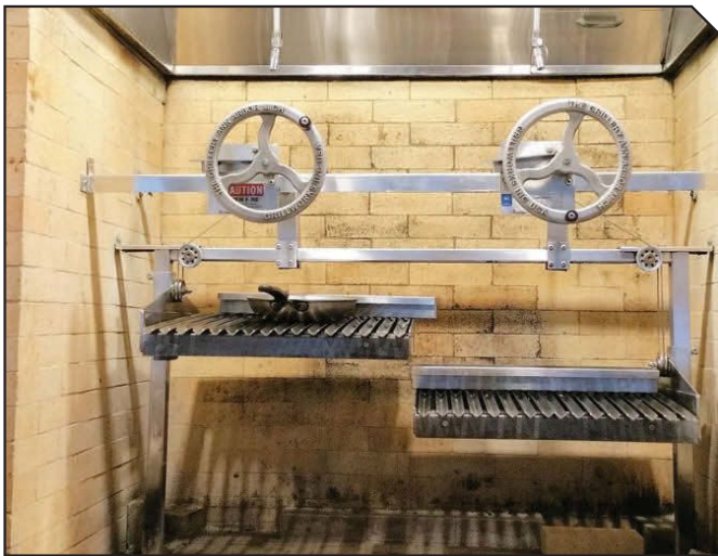
FIGURE 1. Solid fuel cooking alcove and exhaust hood with grease filters removed after post-fire cleanup.
