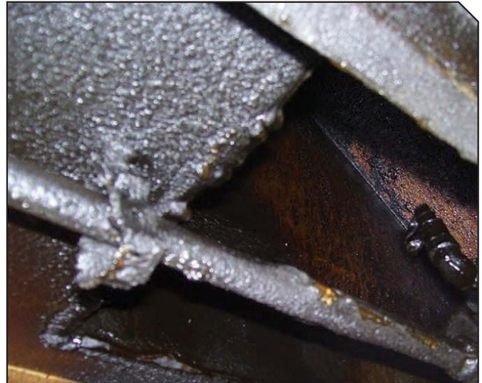
FIGURE 4. Hood plenum without automated hood cleaning.
