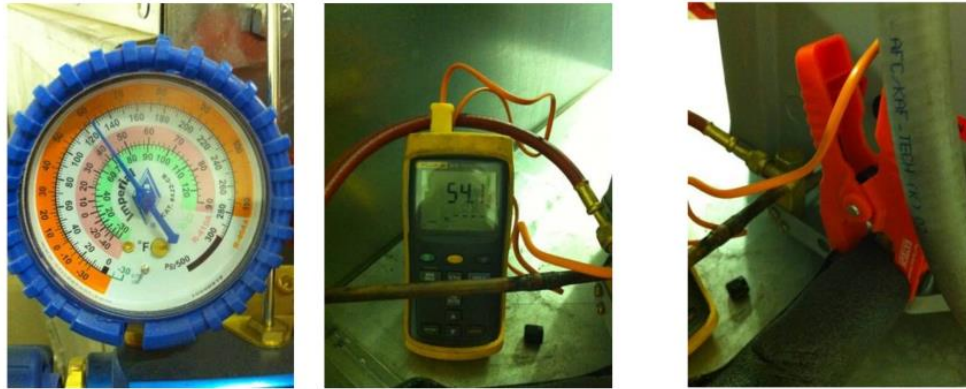
Figure 9 - Gauge Connection/Readings Suction Line
